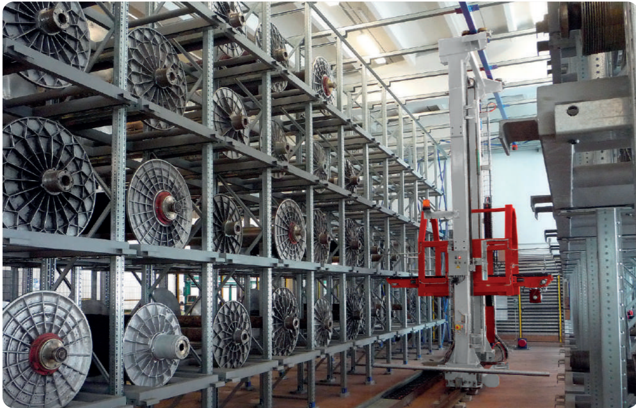
Special automated storage system for rolls of fabric (textile sector)
