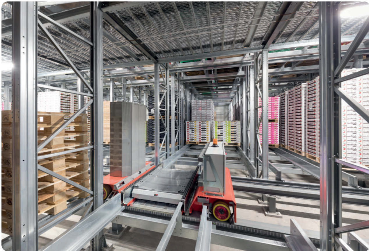
Multi-depth automated storage system with multi-level shuttles (food sector)
