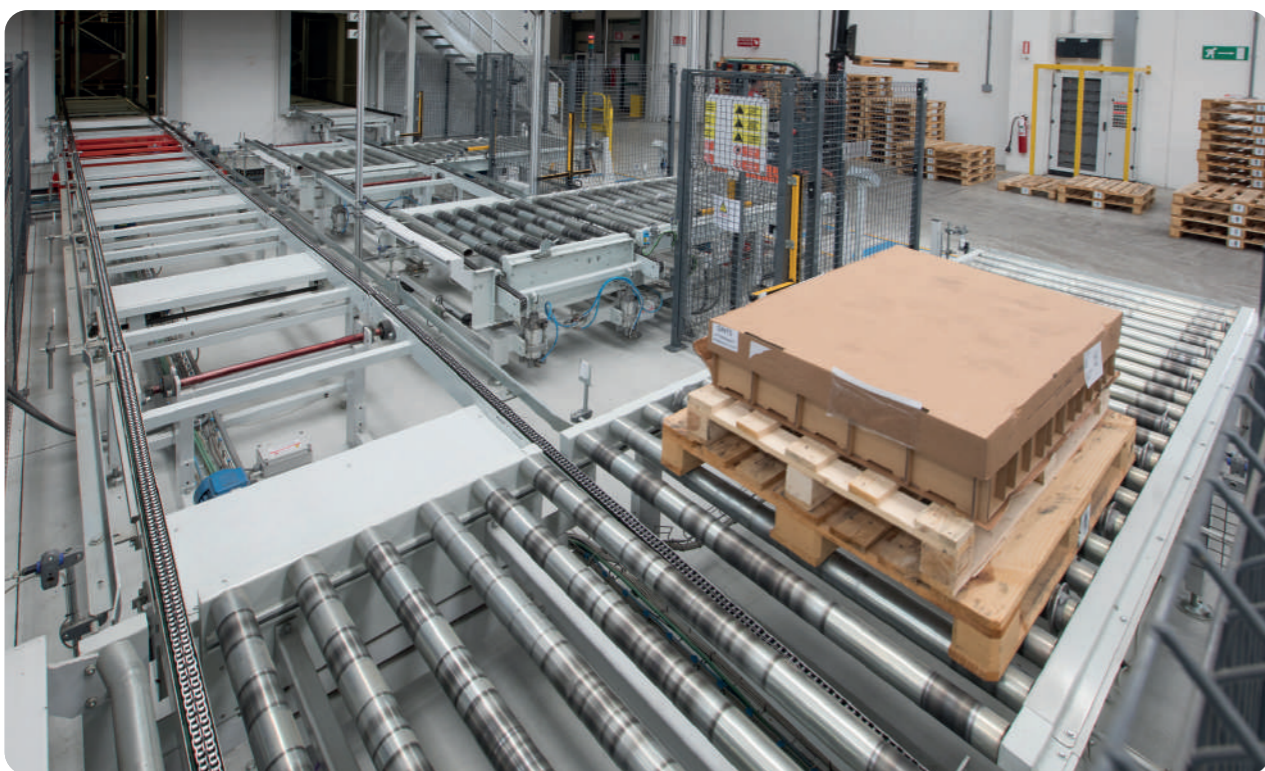
Pallet conveyor line to tilting tables (mechanical sector)
