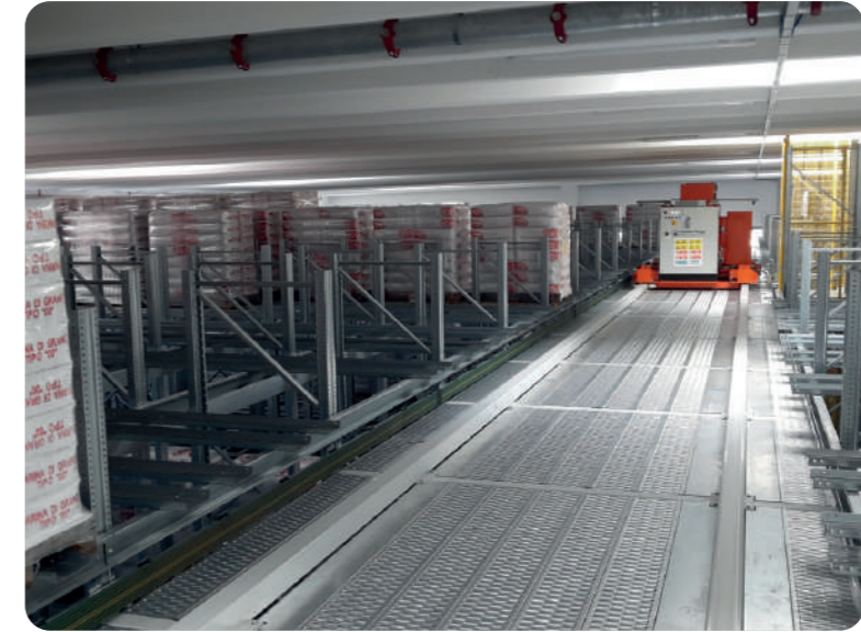
Multi-depth automated storage system with multi-level shuttles (milling sector)
