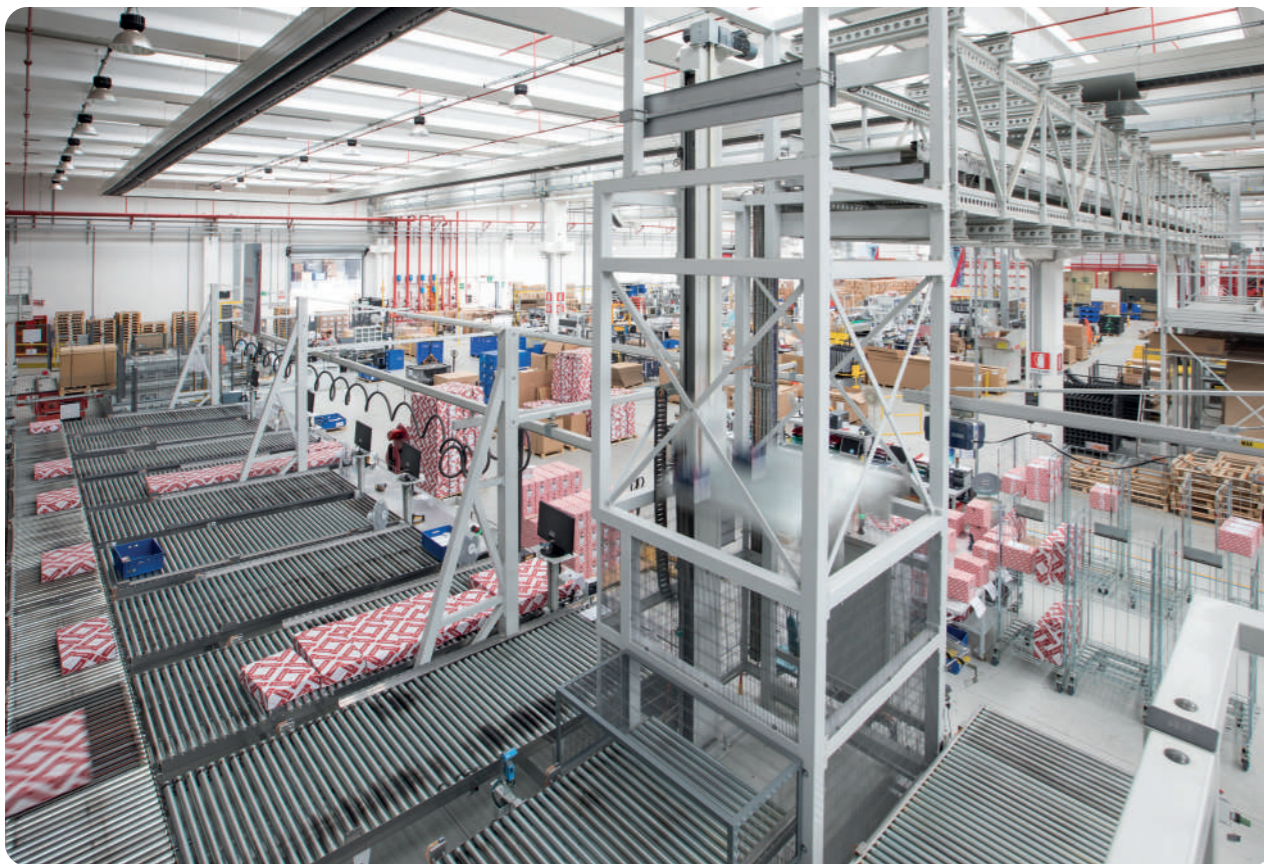
Close-up of lifts for material handling (automotive sector)
